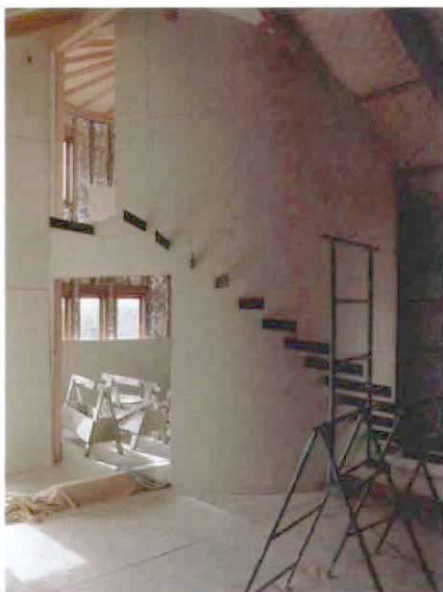
Drywall went on first. Slits were cut in the plywood-and-drywall sheathing materials so that the brackets could be reinstalled from inside the cylindrical room.
